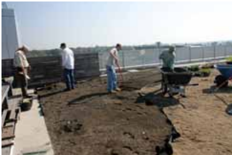
Berkley surveys the installation work on the Clinton Presidential Library green roof project.
